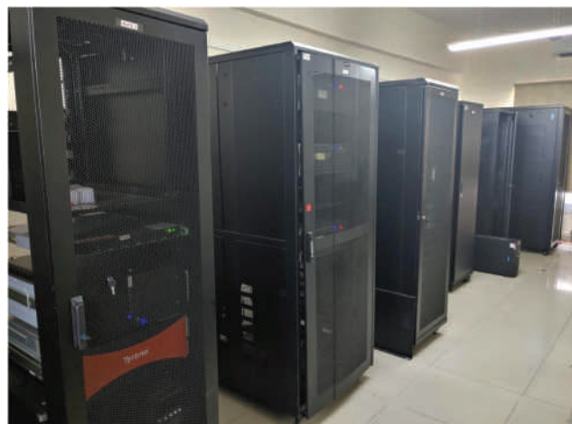
Racks hosting Project Servers/Workstations
