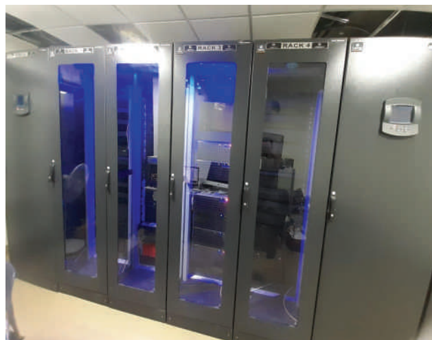
Smart Racks with HPC and GPU clusters
